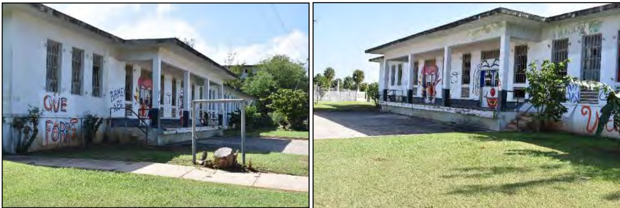
14 Building 508 (Laundry): Photo 6.1-206, left, east side and north front elevations; Photo 6.1-207, right, south rear 15 elevation.
