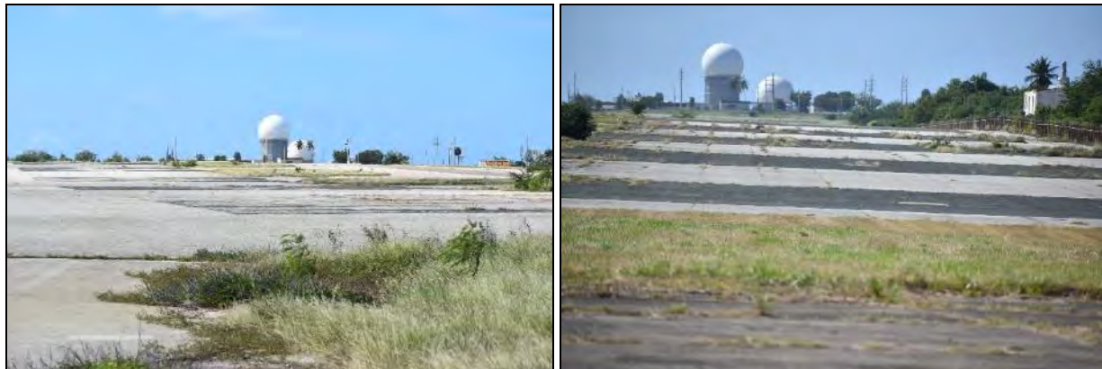
1 Taxiway 2 and Alert Facility Apron: Photo 6.1-425, left, ground-level views looking west from western end of apron; 2 Photo 6.1-426, right, ground-level views looking east from eastern end of apron.
