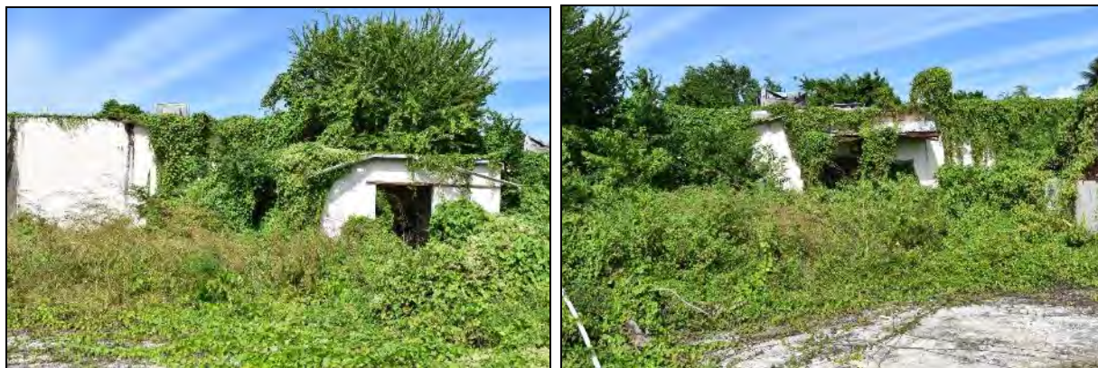
22 Building 1128 (Armaments and Avionics Shop): Photo 6.1-374, left, western third of S front elevation; Photo 6.1-375, 23 right, central third of S front elevation
