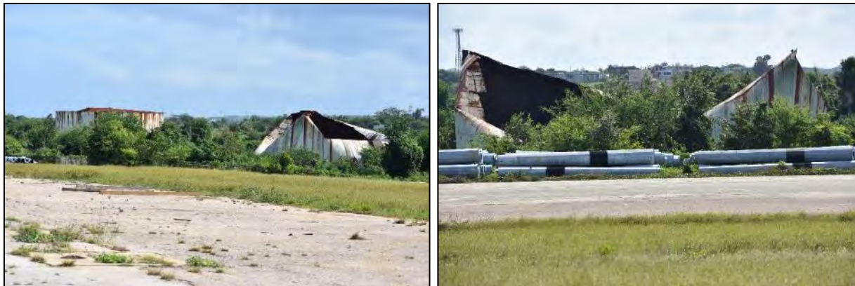
1 Tank 1214 (Fuel Storage Tank): Photo 6.1-474, left, looking southeast at Tanks 1215 and 1214, left to right; Photo 6.1- 2 475, right, looking south at Tank 1214.
