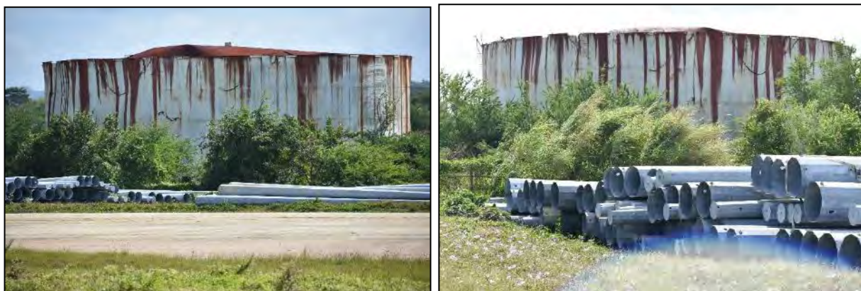
14 Tank 1215 (Fuel Storage Tank): Photo 6.1-476, left, looking south at tank, left to right; Photo 6.1-477, right, looking 15 southeast at tank.
